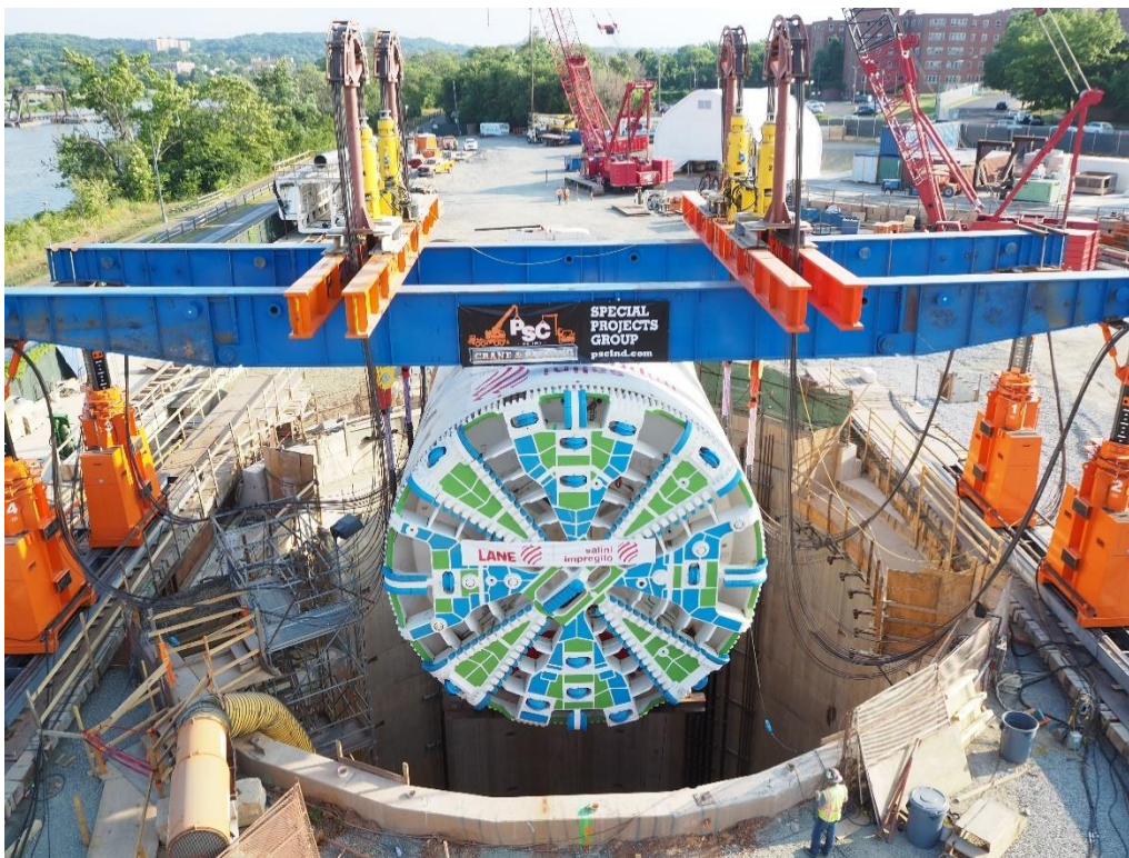
Figure 8. Example of a Large-diameter TBM Cutterhead and Shield Being Lowered into a Main Work Shaft
