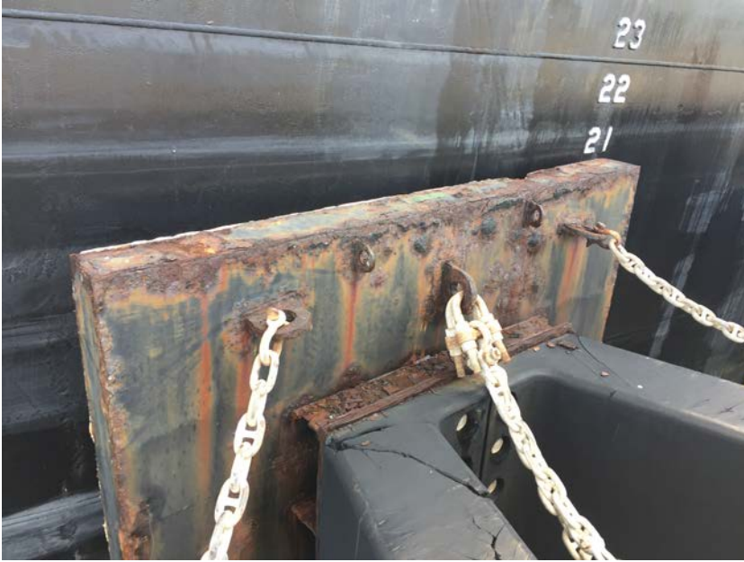
Corroded Ship Breasting Structure Fender Panel and Damaged Rubber Element
