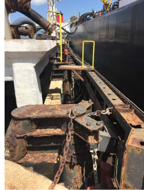
Corroded and Misaligned Barge Fender Panel Systems
