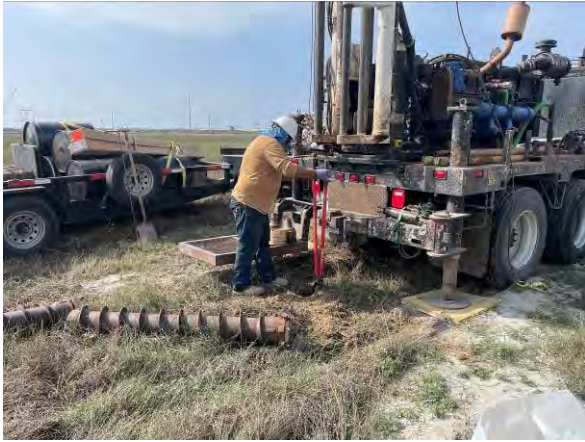
Photo 1 Clearing of boring location DMMU-1-1A / DMMU-2-1A with posthole digger to 5 feet bgs.
