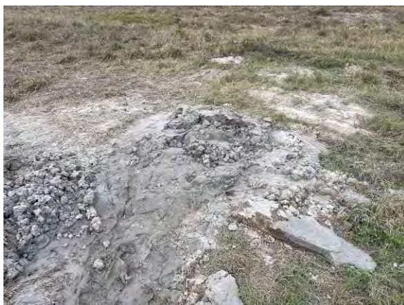
Photo 11 View of typical land-based boring following grouting with cuttings and bentonite slurry.
