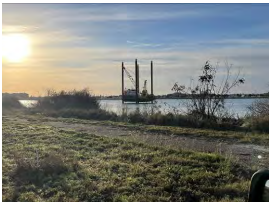
Photo 17 View of boring location DMMU-7-4B prior to advancement of boring, facing southeast.
