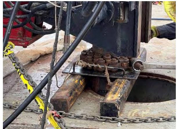
Photo 20 View of lift boat moonpool where sediment samples obtained utilizing sonic drill rig.
